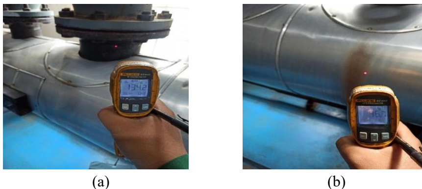
Gambar 3. Temperatur in-situ pipa steam header (a) Tanpa insulator, (b) Tertutup insulator
