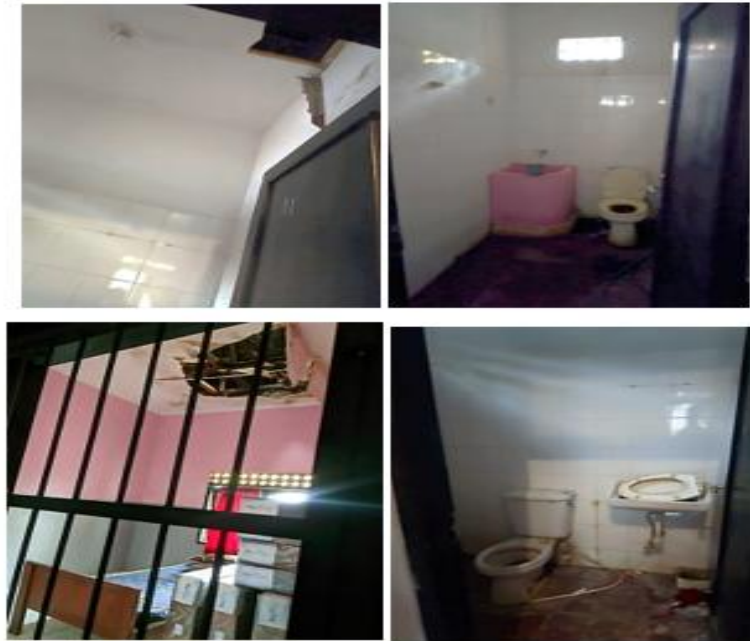
Figure 2. Damaged Facilities and Infrastructure
