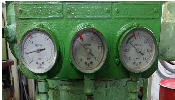
Figure 3.2 Compressor pressure gauge decreases
