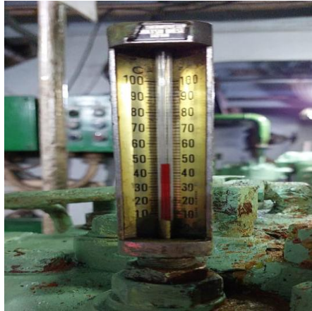
Figure 3.1 The Compressor Cooler is experiencing overheating
