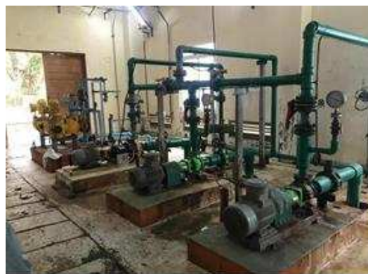
Gambar 7. Continous Dosing Pump
