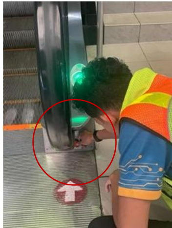
Figure 4. Manual Operation of Escalator (Source: Author documentation, 2024)
