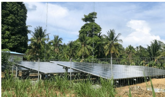
Figure 2. Solar Power System of Miang Island Village
