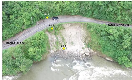
Figure 2. Landslide on the Pagar Alam – Tanjung Sakti Road at KM 320+500
