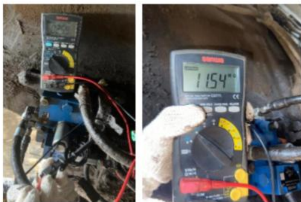
Figure 4. EPC Hoist HSOL Solenoid Measurement
