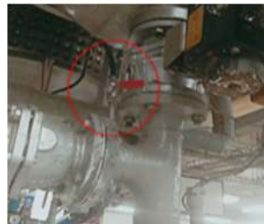
7. Open the thinner bubbling valve for the T-valve cleaning process.
