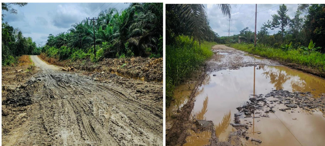
Figure 3. Road damage in Sabung Village (January 2024).
