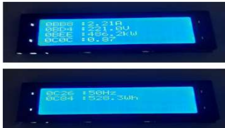
Figure 9. Energy Meter Testing
