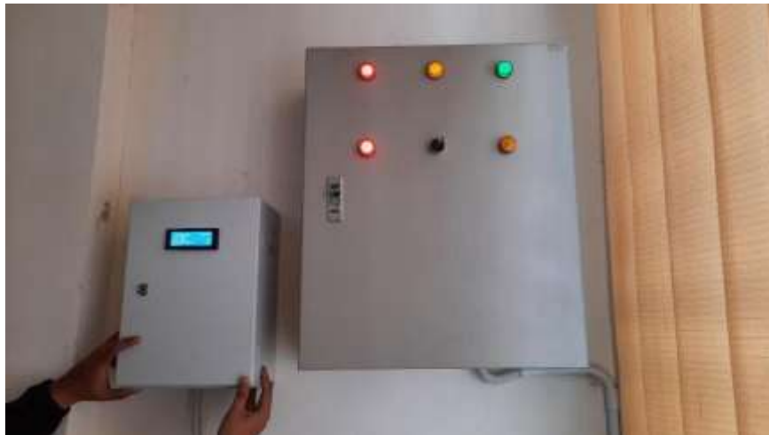
Figure 7. Overall Tool (SiSCE control panel)
