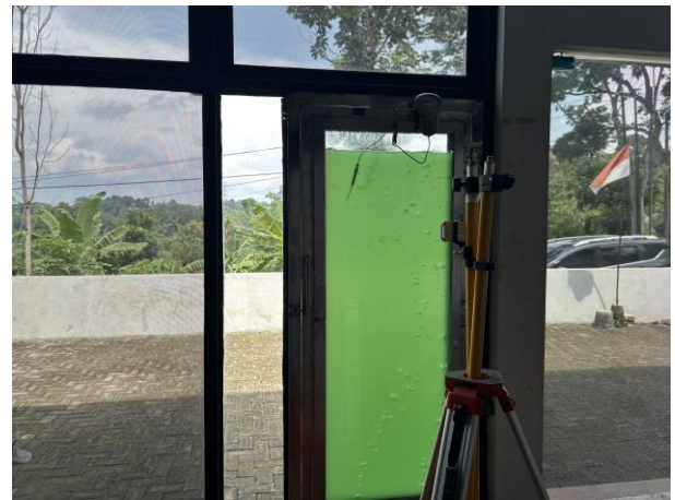
Fig 3. Installation view of the photobioreactor façade system, representing the baseline niche innovation in this study.
