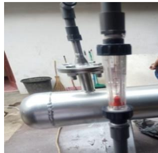
Figure 1. Seawater flowmeter and seawater inlet line.
