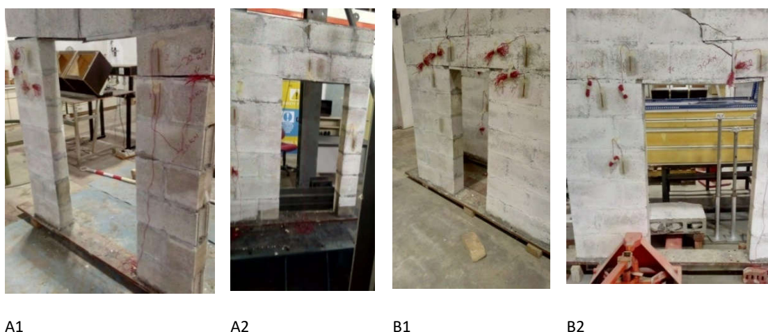
Figure 3 The cracking patterns of wall panels A1-B2.
