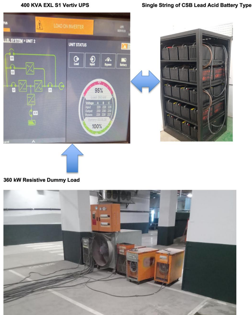
Figure 12. Resistive Dummy Load with Lead Acid Battery Type connected to a 400 kVA Vertiv UPS during testing
