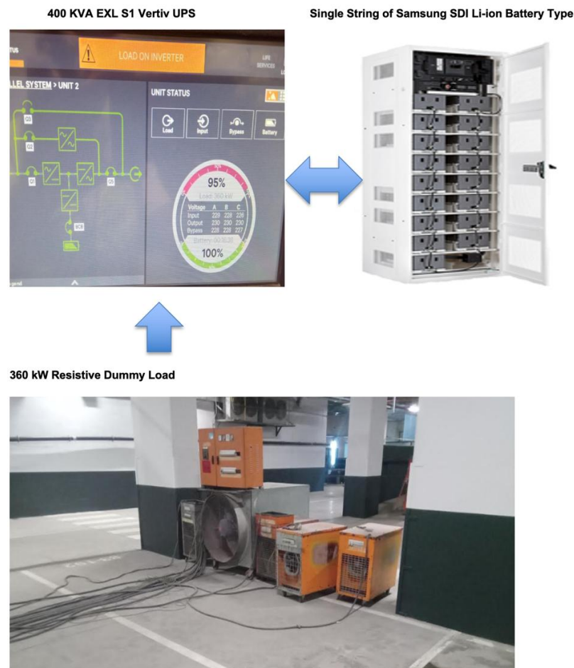
Figure 11. Resistive Dummy Load with Samsung SDI Battery connected to a 400 kVA Vertiv UPS during testing
