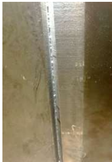
Fig. 4. Welding Seam Before Back Gouging
