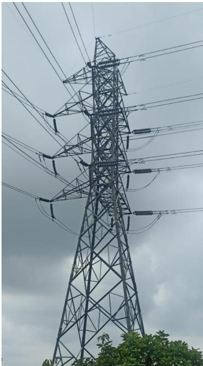
Gambar 2.1. Tower TEA 58A SUTT 150kV Sindang Jaya - Suvarna
