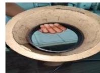
Figure 5. Existing core plug (before repair)
