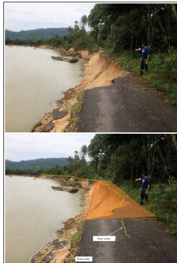
Figure 7. Sketched area of the broken road due to the occurrence of a landslide, also clearly observed the breakdown of the tar road at the bottom of the slope.
