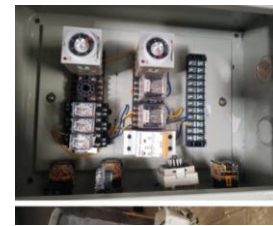
Fig. 6. Filling Machine Control Panel
