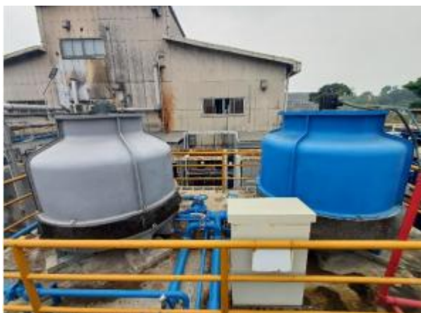
Gambar 3. Tipe induced draft cooling tower
