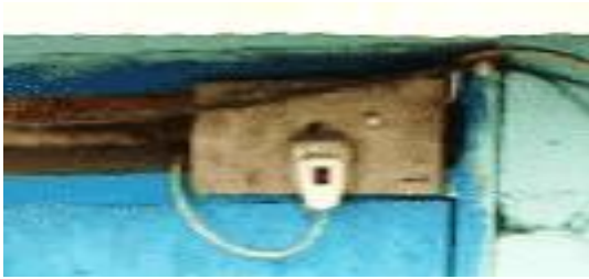
Figure 6. Sockets Outside The House Without Canopy or Protector
