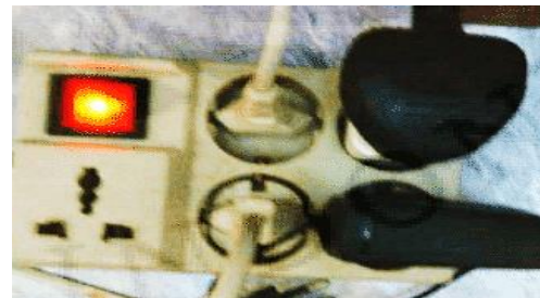
Figure 5. The Electrical Circuits Being Used Simultaneously
