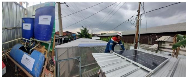
Fig. 4. Environmentally Friendly Water Filtration System (SITIRTA) with Solar Panels
