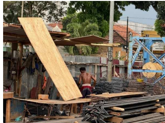
Figure 1. Workers Do Not Use PPE While Working
