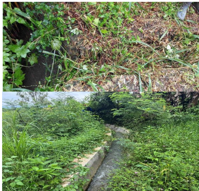
Fig. 7. Condition of the Irrigation Channels in Bdr. Imang
