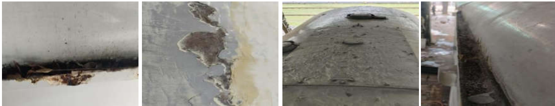
Fig. 1. Corrosion on Mild Steel Train Roofs
