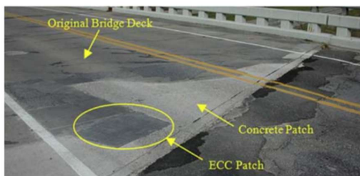
Figure 6 Successful Study of ECC Application to Michigan Bridge Deck (Boughanem et al., 2013; Yildirim, 2018; Yin et al., 2019).
