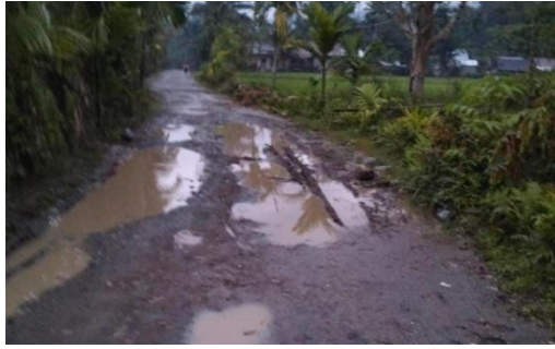
Figure 1. Severely Damaged Road Conditions
