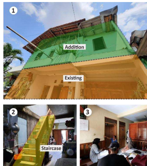
Figure 4. (1) Vertical addition above the existing mass in case 2; (2) Proper staircase connecting the first and second floors; (3) Interior space constructed with appropriate dimensions and materials
