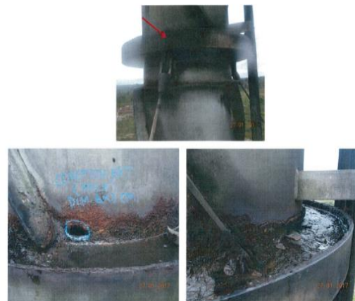
Figure 1. Hole due to External Corrosion (circular) with dimension 2.4" length and 1.2" width at 18.00 o'clock position on flare stack (riser) of connection Ring area of F-2900A. The nominal thickness of flare stack (riser) is 30" OD x 0.250" thick.
