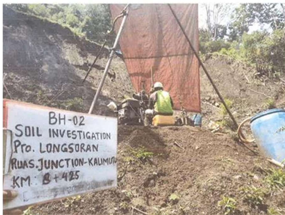
Figure 2 Slope Failure Conditions on STA 8+425 (Source: Sasarari et al. , 2024a)
