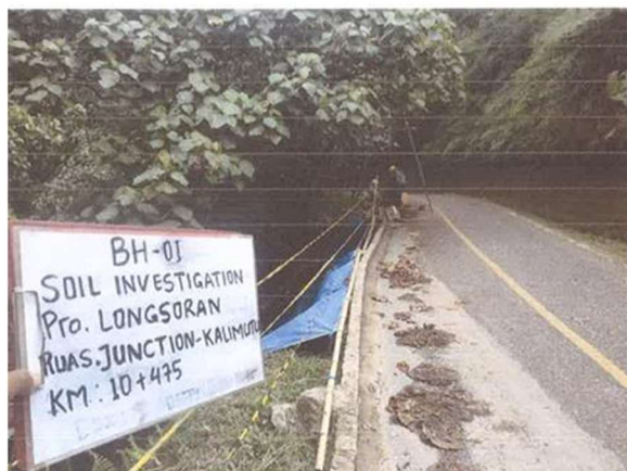
Figure 3 Slope Failure Conditions on STA 10+475 (Source: Sasarari et al. , 2024a)
