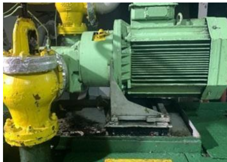
Figure 1. Lubricating Oil Standby pump on board of MT. Klawotong Source : Researcher's documentation (2023)
